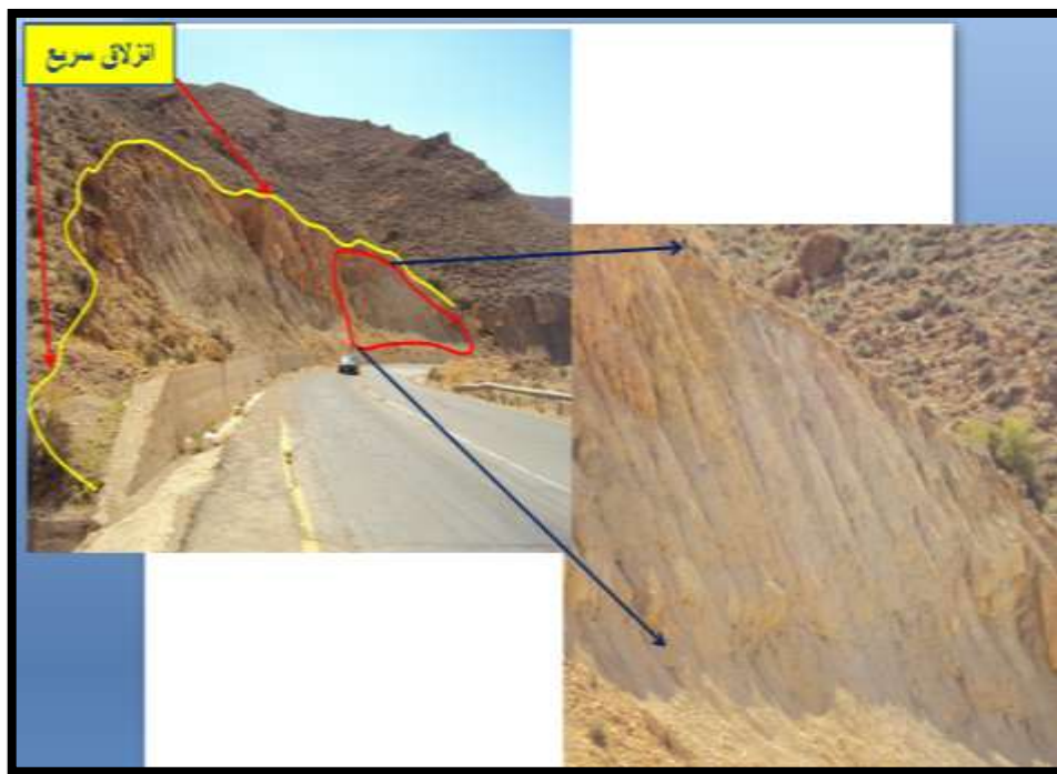
Figure (11): Shows the landslide at the first site in the Al-Labib area.
