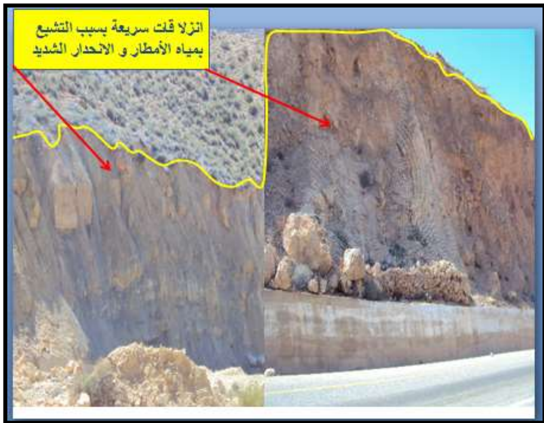
Figure (12): Shows the second site in the Al-Labib area, illustrating the rapid ground failure caused by the steep slope.
